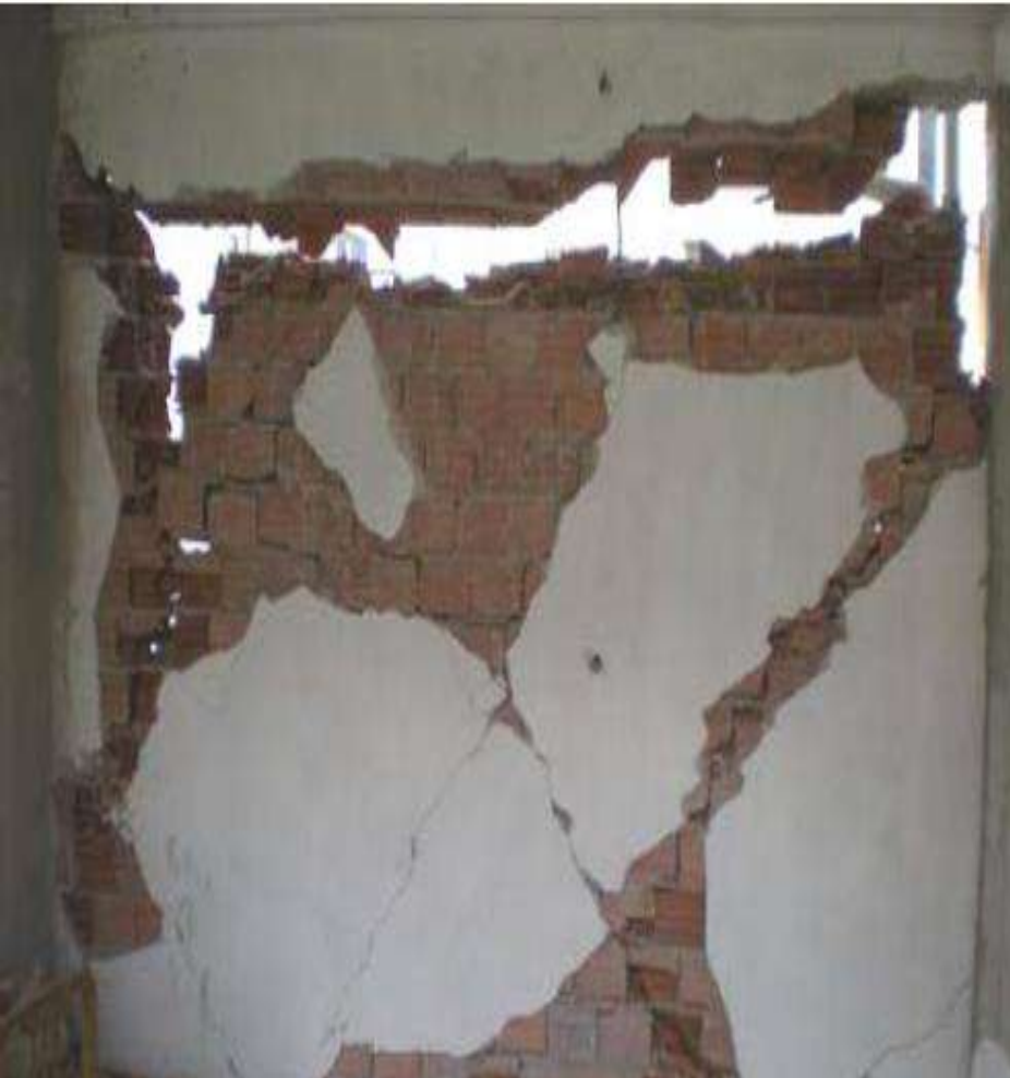
Kutahya Earthquake, Turkey, May 29, 2011
