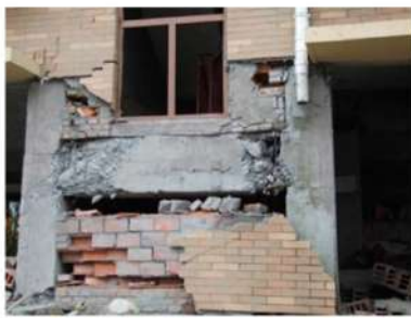
(b) Damage to two sides of the landing beam
