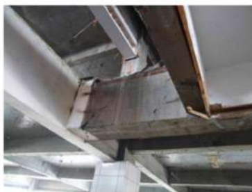
(e) Unidirectional shear cracking on "short beam"
