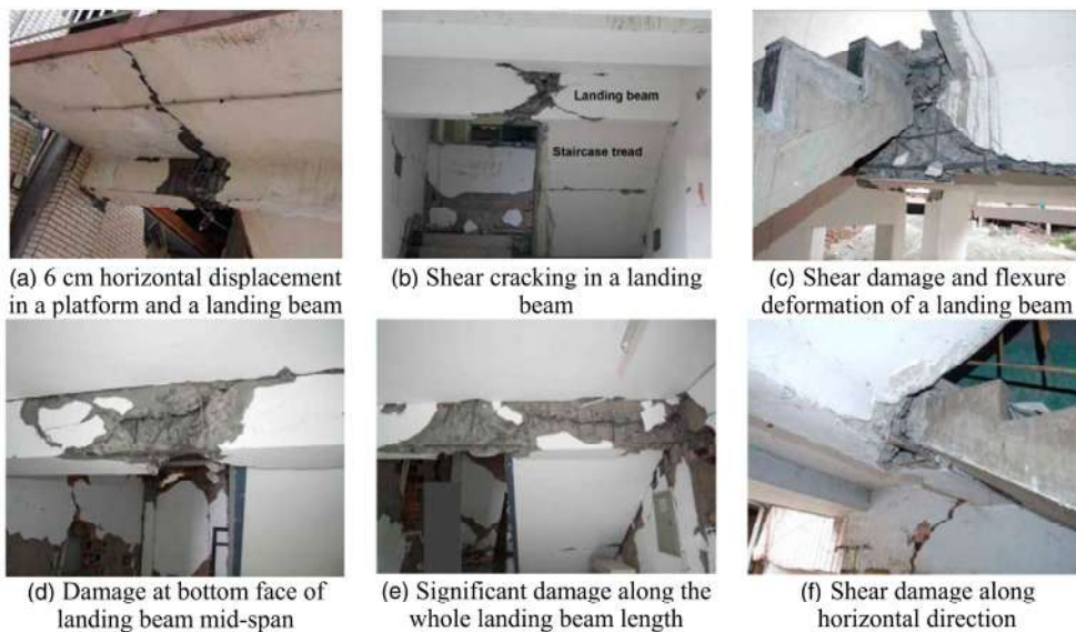
Fig. 9. Observed failure of landing beams: (a) 6-cm horizontal displacement in a platform and a landing beam; (b) shear cracking in a landing beam; (c) shear damage and flexure deformation of a landing beam; (d) damage at bottom face of landing beam midspan; (e) significant damage along the whole landing beam length; (f) shear damage along horizontal direction
