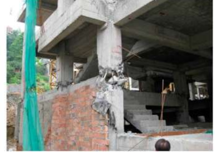
(b) Failure of joints
