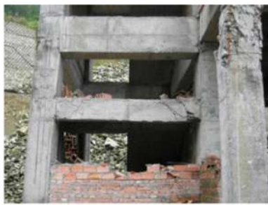
(a) Shear cracks on two sides of the landing beam
