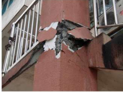
(a) Concrete spalling in slab-column joint
