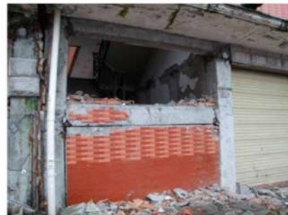
(c) Vertical cracks on two sides of landing beam
