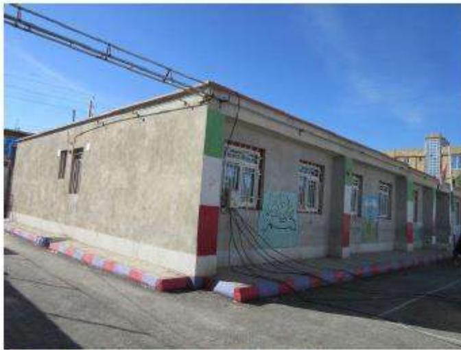
a) The building with few hairline cracks on some of the walls
