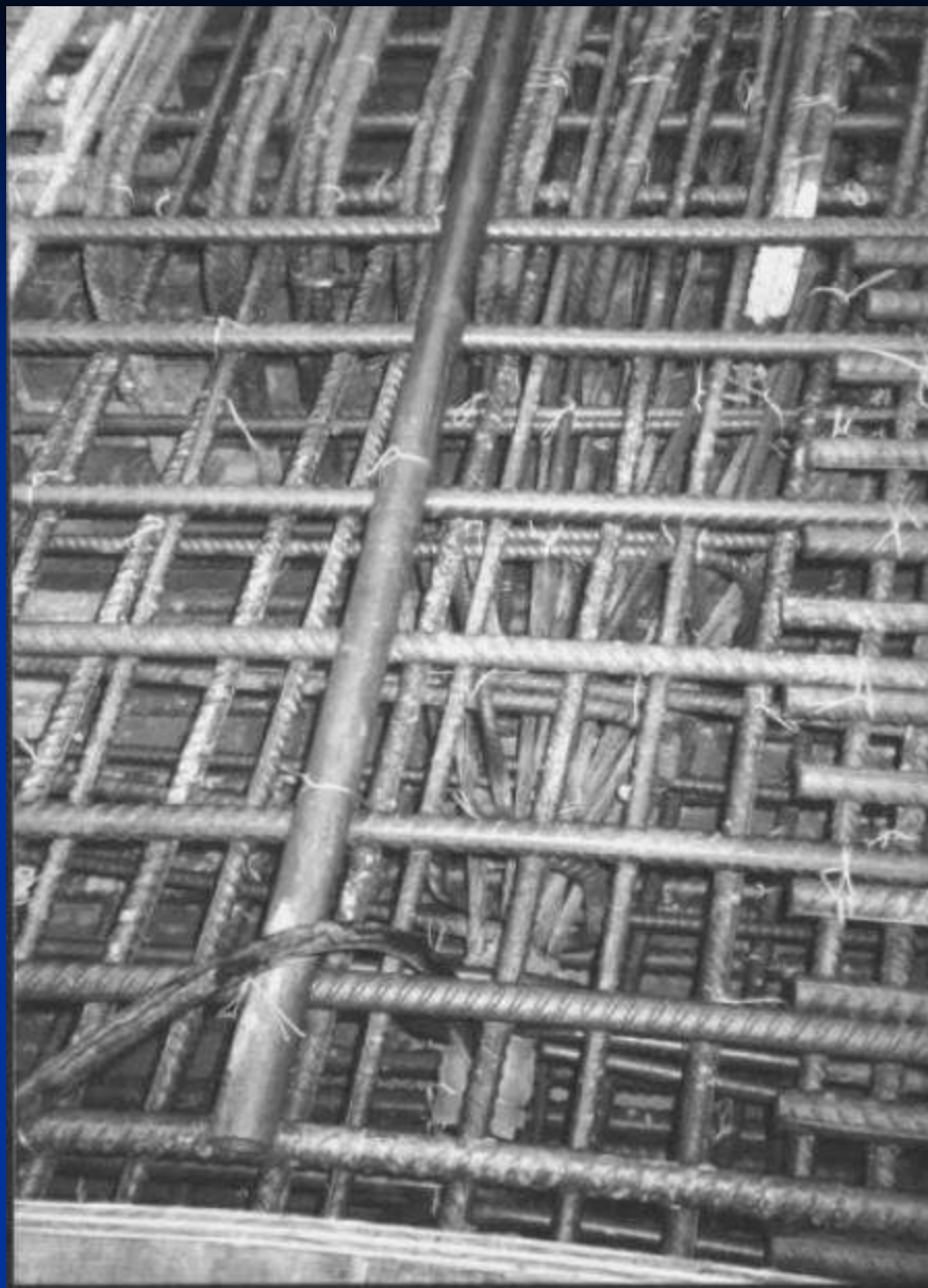
Fig. 2. An example of congested reinforcement: an ideal application for SCC (Mott MacDonald Ltd)
