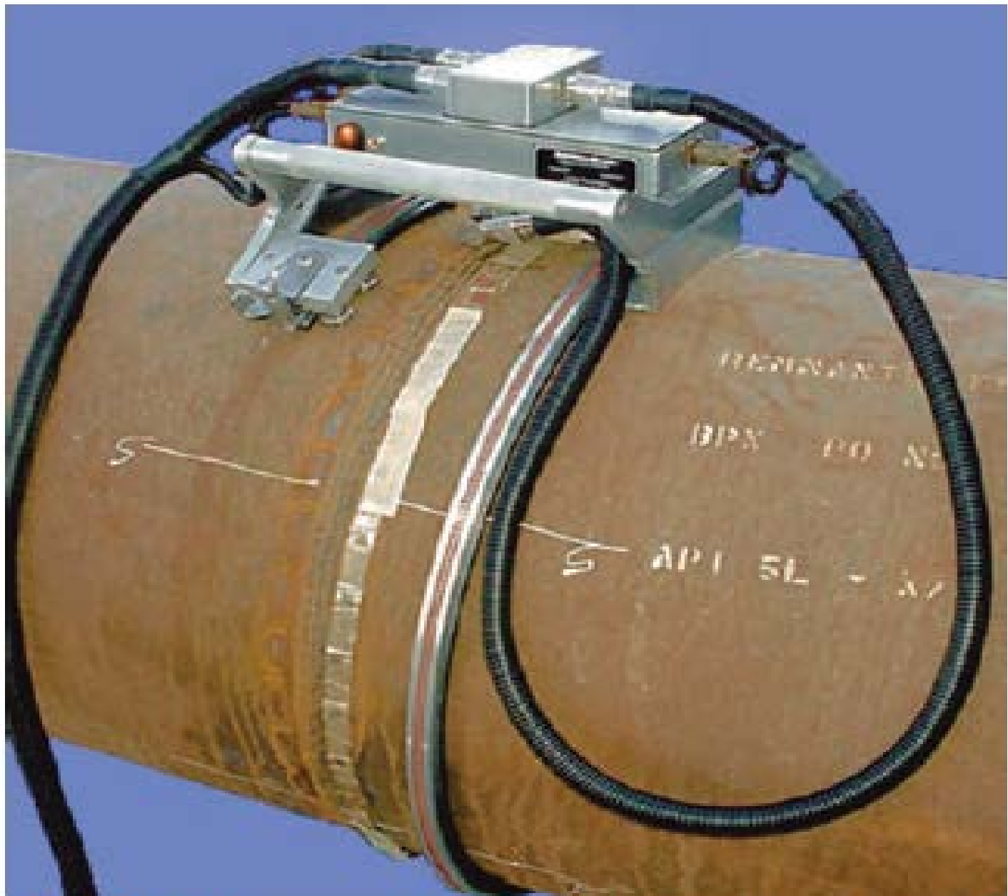
FIGURE 23-40 Preparing to test the quality of a weld on a pipe using X-ray equipment. CMOS X-Ray
